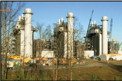
HRSG exhaust silencers installed at Tenaska for GE Frame 7FA turbines
