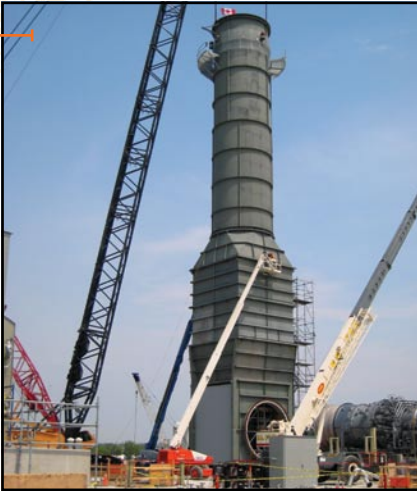
One of two 150 ft tall exhaust stacks supplied by ATCO/HK for a 550 MW station in Ontario, Canada.
