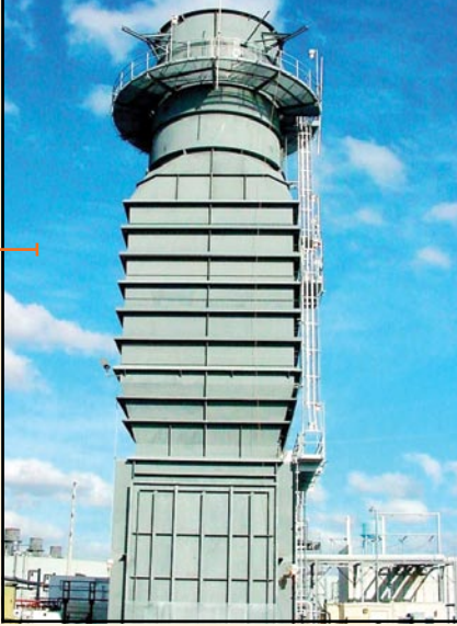
GE Frame 7FA exhaust system retrofit to meet critical low-frequency noise limitations during start-up and at base load
