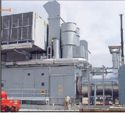
ATCO/Higgott-Kane model anti-icing system installed on a GE LM6000 turbine
